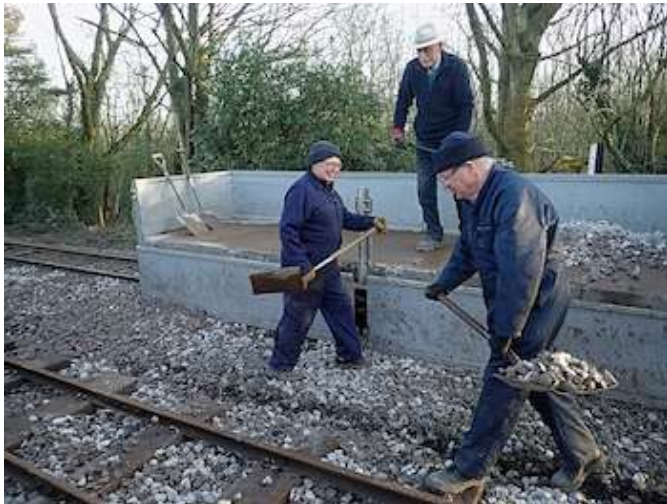
The closed season for traffic is very much open for maintenance and upgrade work. Here the sleepers and ballast are being renewed at Delph station.
