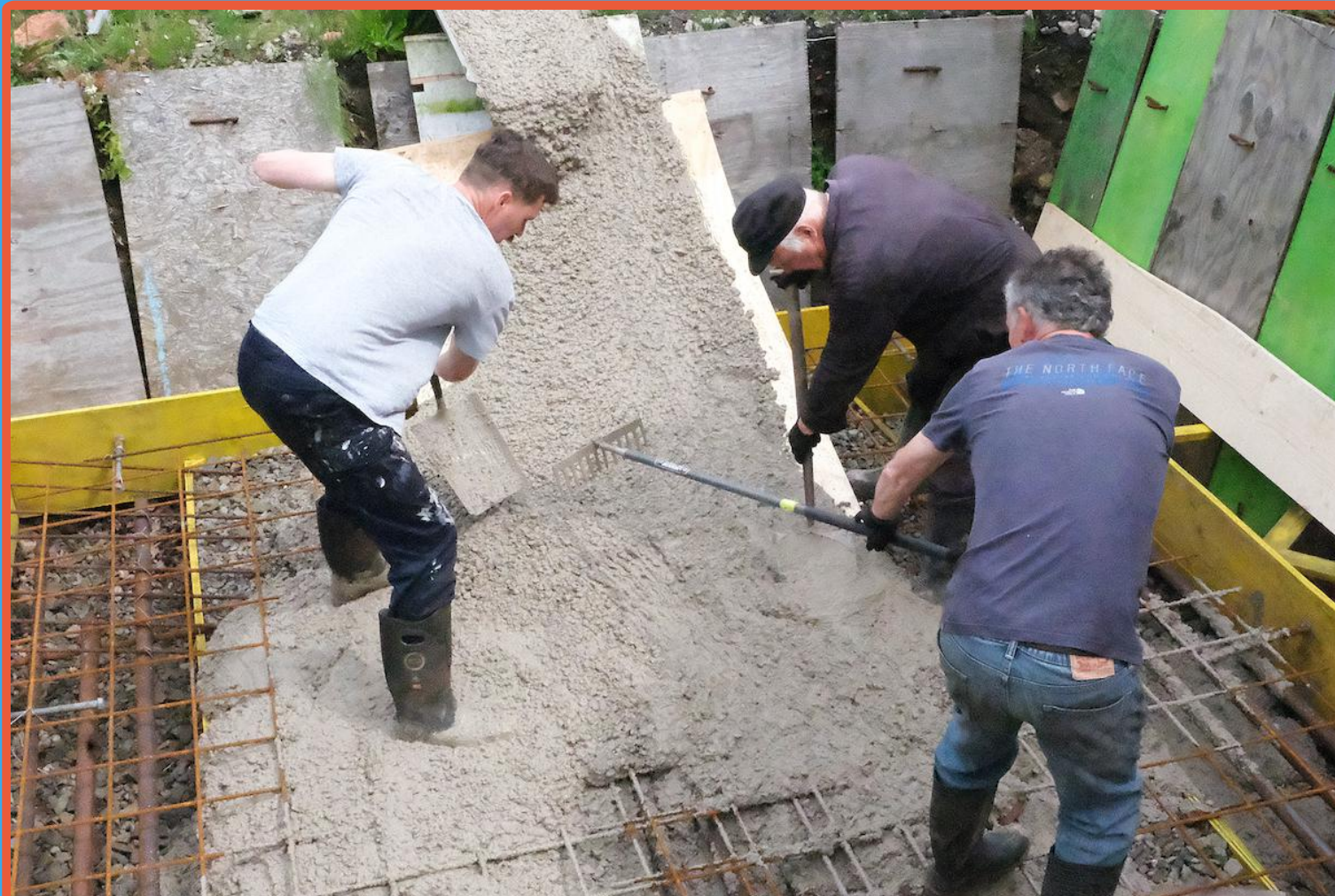
Sometimes the fun is almost too much. Simon, Paul and Mike get to shovel and rake several tonnes of wet concrete, to form the base of the new ash pit.
