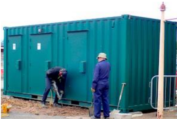
Andy (1) and Keith prepare the trench for some concrete in front of the new toilet block...
